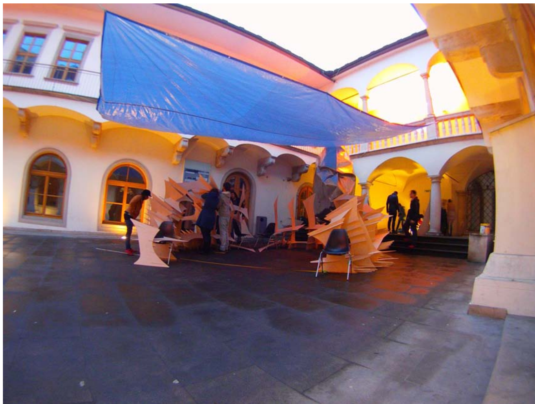
Assembly of the structure at the courtyard of The House of the Lords of Kunštát in Brno
